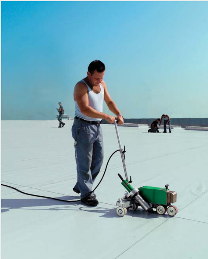
With the VARIMAT V walk welder, Columbia River Roofing was able to weld 22,000 to 25,000 square feet per day.
