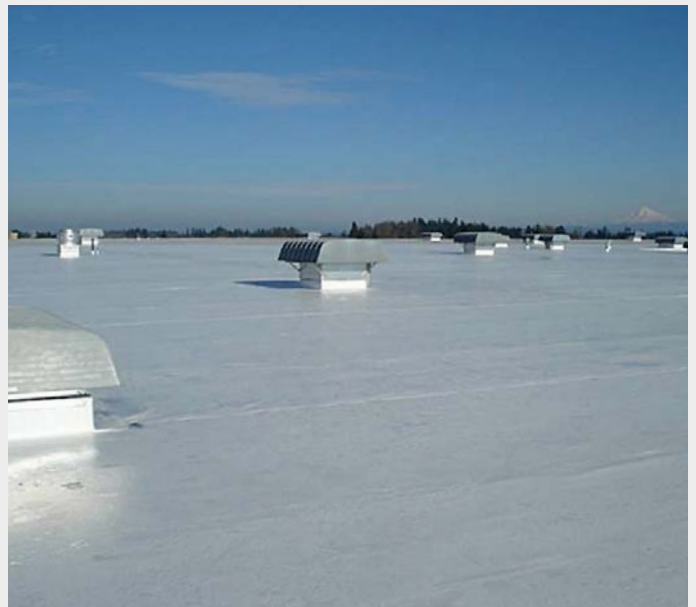
Columbia River Roofing was able to complete the new Food Services of America roof in less than two months due to the reliability and efficiency of Leister tools.
