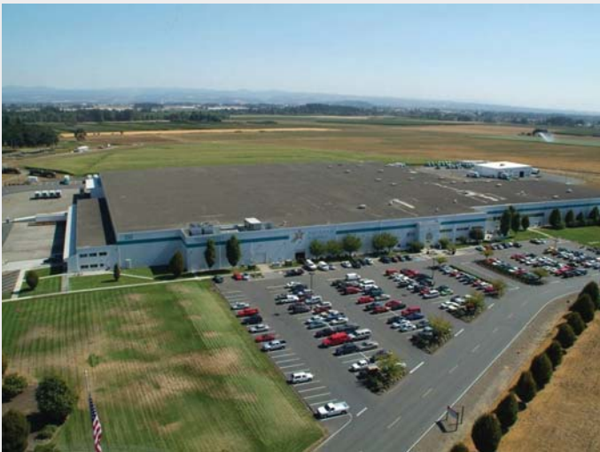
The massive 420,000-square-foot ballasted roof atop Food Services of America's Woodburn, Ore., distribution center had seam failures tearing as fast as 50 feet per week.
