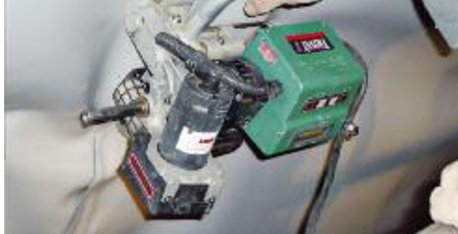
TWINNY T, with convenient cross-handle, at work overhead welding in a tunnel.
